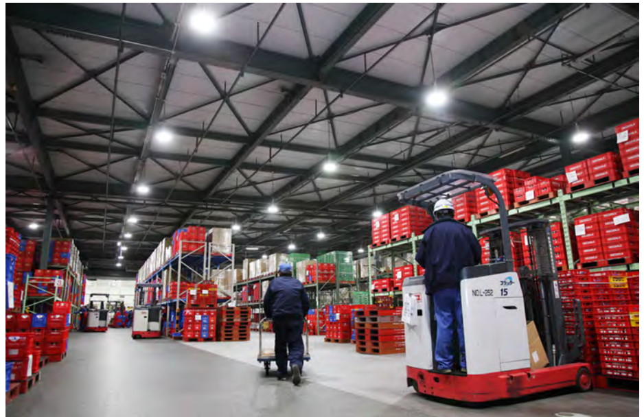
MEGMILK SNOW BRAND Co. Ltd's Noda facility runs 24 hours a day. The LED lights are dimmed in unoccupied areas to maximise energy savings whilst also ensuring employee comfort and safety.
